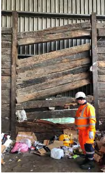
Above – photograph of damaged sleeper wall
